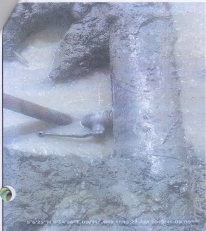
Figure 1: Installed Valve on the pipeline.
